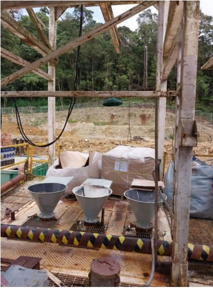
Emergency shower was not clearly visible
