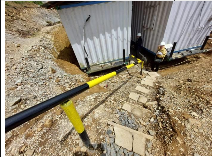
Proper and safe walkway provided
