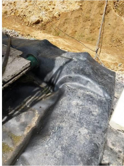
Bund walls need repair
