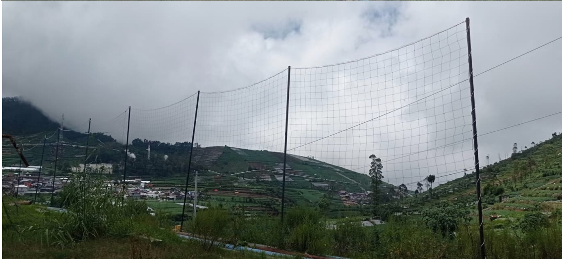
The contractor completed the net construction around Pad 30, which functioned as the Pawuhan Community's soccer field.
